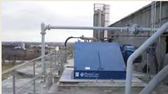
CPV Multiple cement silos 4,800 cfm
