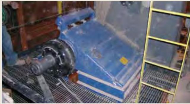
CPV Bucket elevator 1,200 cfm
