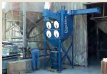
DFO Concrete roof manufacturer 3,000 cfm
