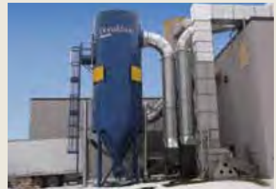
RF Cabinet shop 48,500 cfm
